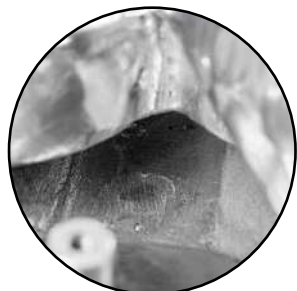
Open area under the plenum
