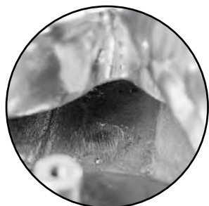
Open area under the plenum
